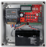
Deep Cycle 12Ah Battery 20W.
