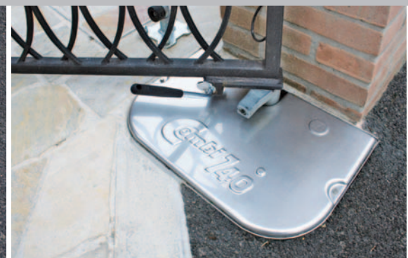
Detail of the opened gate with emergency release device
